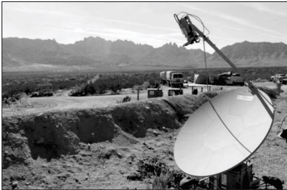
Figure A-14. SIPRNET/NIPRNET Access Point
