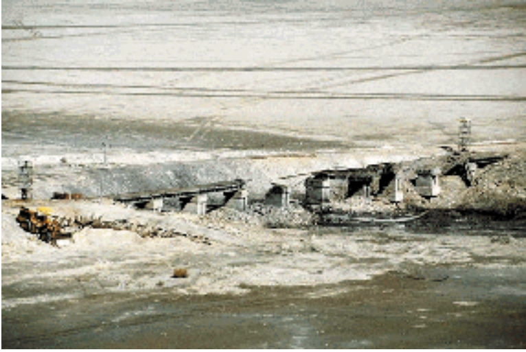
A railroad bridge near the Arramaylan refinery damaged by Allied bombing during Operation DESERT STORM.
